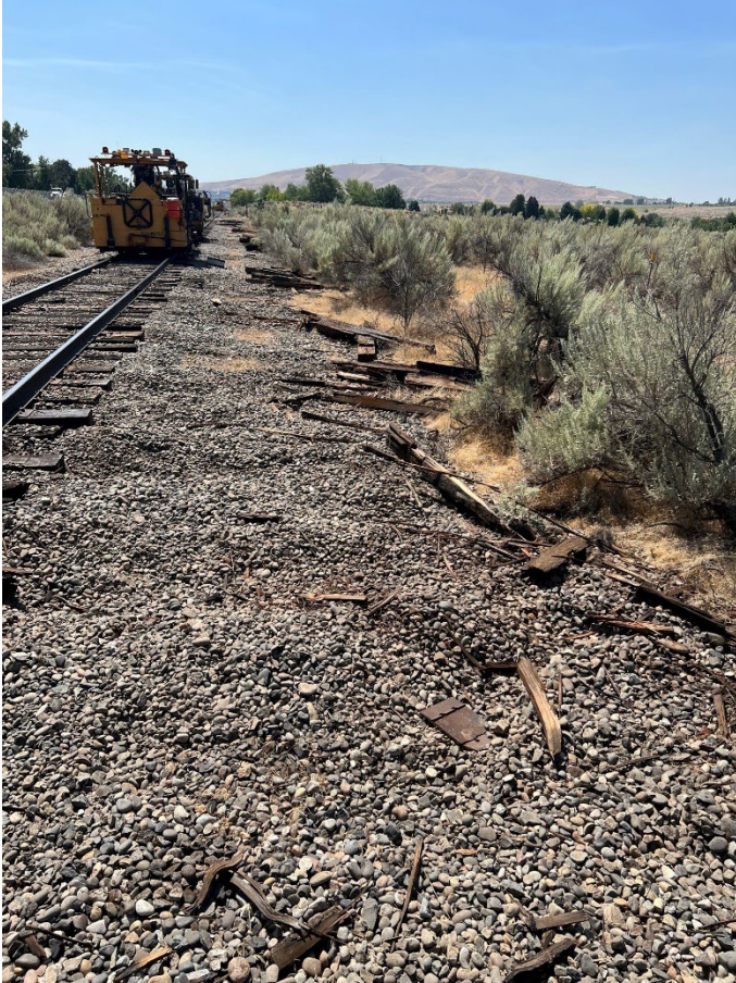
Old removed ties and disturbed ballast
